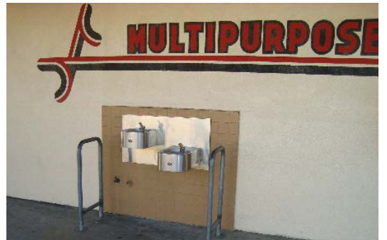
Interior/exterior of buildings need to be repainted.
