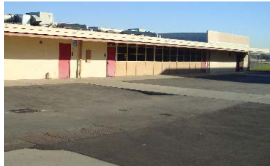
Existing paving in poor condition throughout campus.
