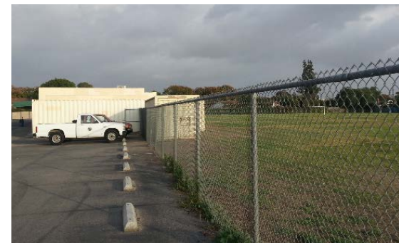
Need to replace fencing throughout.
