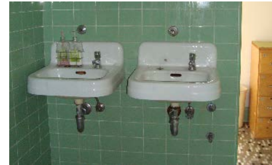
Restrooms are in need of upgrades.
