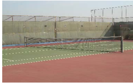
Tennis courts need resurfacing.
