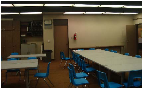
Need to improve lighting.
