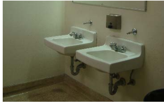
All restrooms need renovation.
