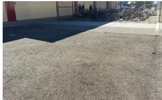
Campus-wide paving is in poor condition.
