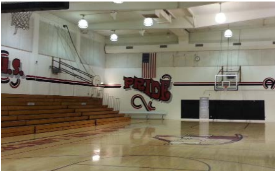
Gym floor and bleachers need to be replaced.
