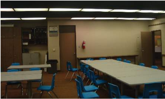
Need to improve lighting.
