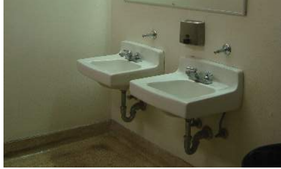
All restrooms need renovation.
